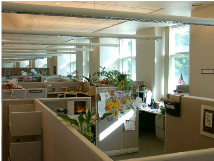
Figure 6: Luminaire arrangement on top floor of CSC building with skylights Note luminaires perpendicular to windows, top floors only.
