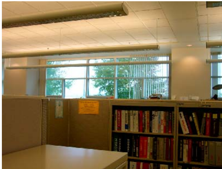
Figure 4: Direct/indirect luminaire and recessed downlights in CSC building
